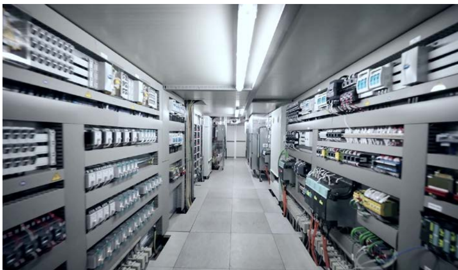
Electrical control equipment built in thermal-insulated In-Box Container complete with heat exchangers for indoor temperature control (air conditioning)
